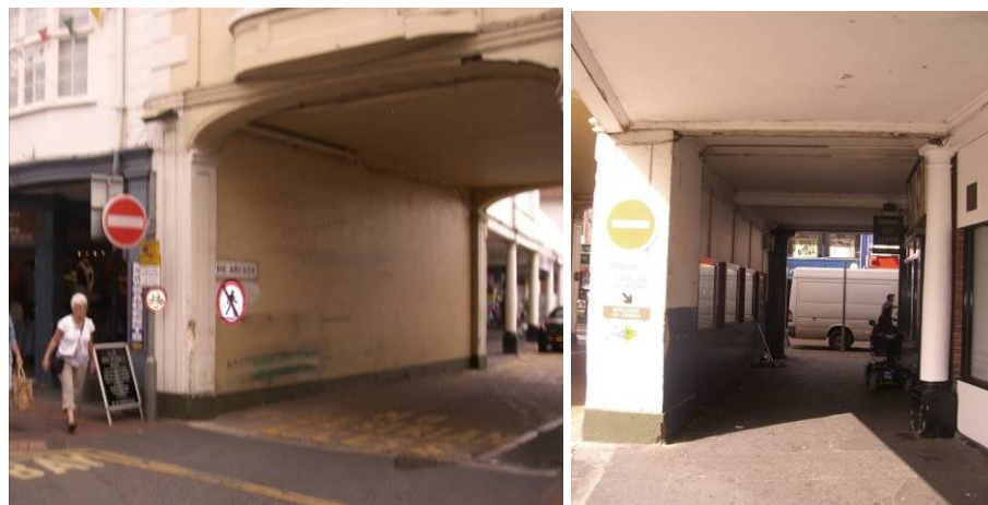
Figure 5.5 – Poor entrance to ferry terminal
